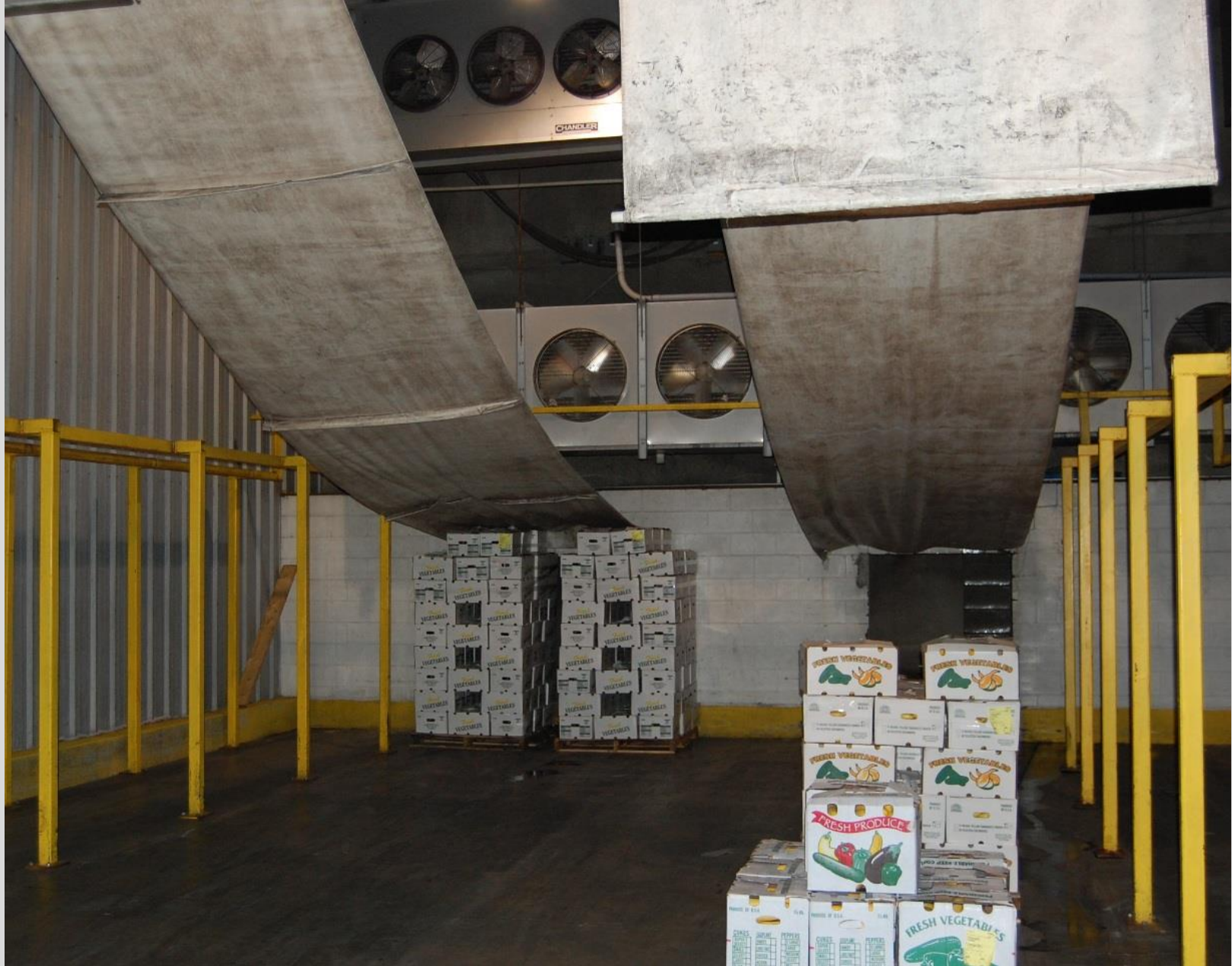
A typical commercial tunnel-type forced-air cooling system in Georgia
