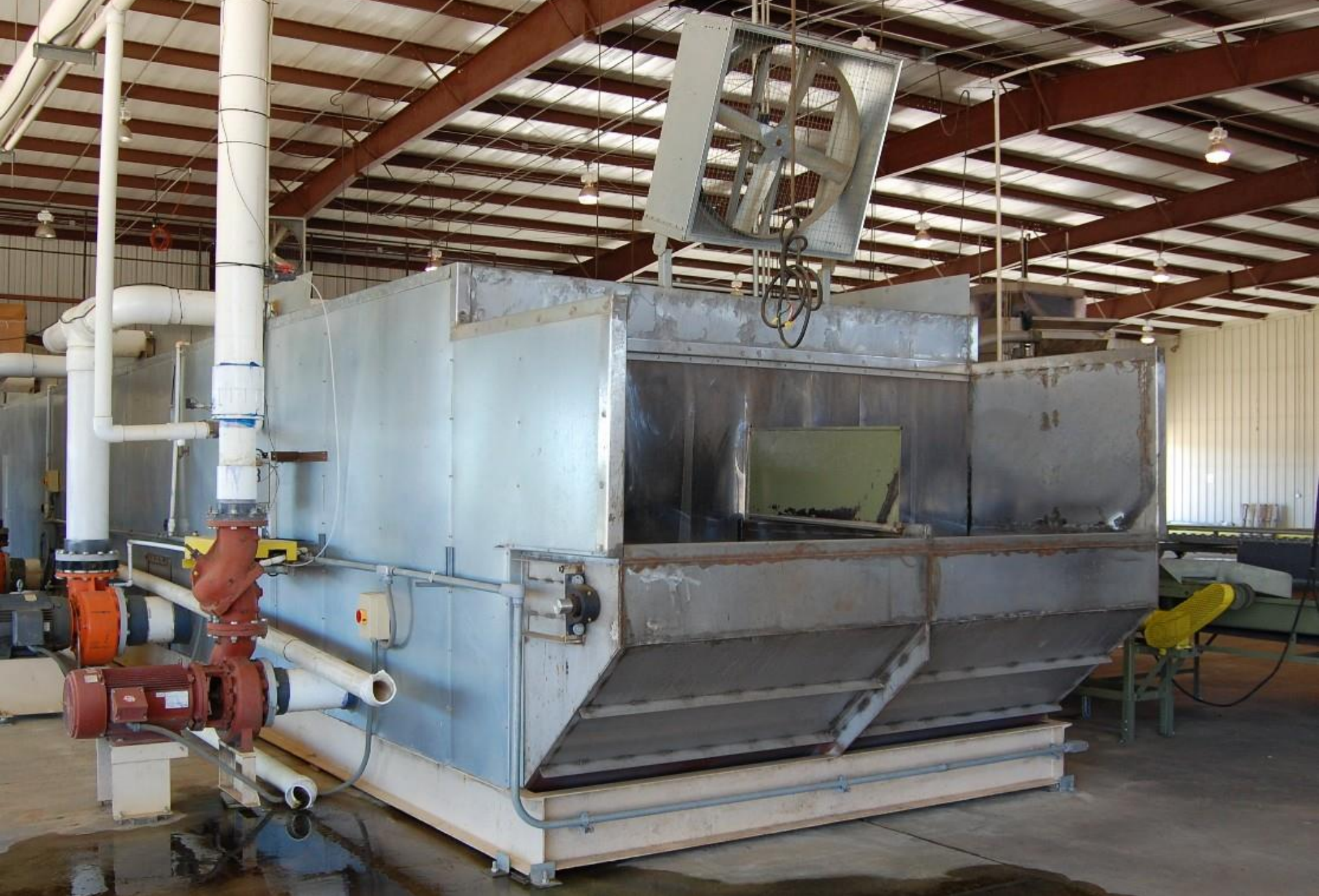
A commercial hydrocooler in Georgia
