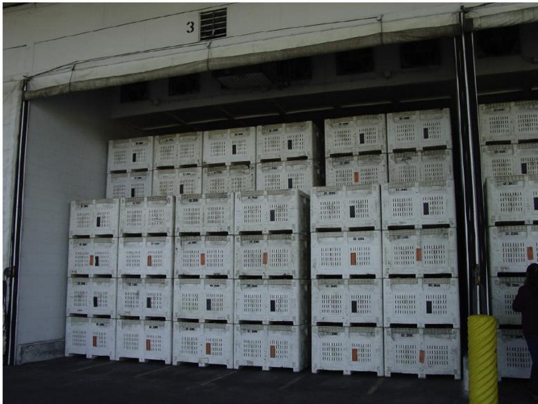
FIG. 9.37 Citrus degreening room.
