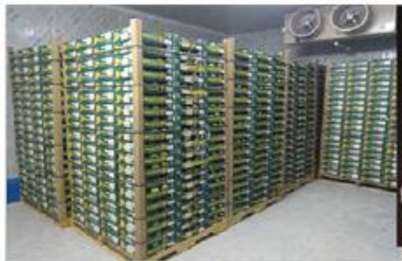
Shipment Ready Pelletized Boxes in Cold Room
